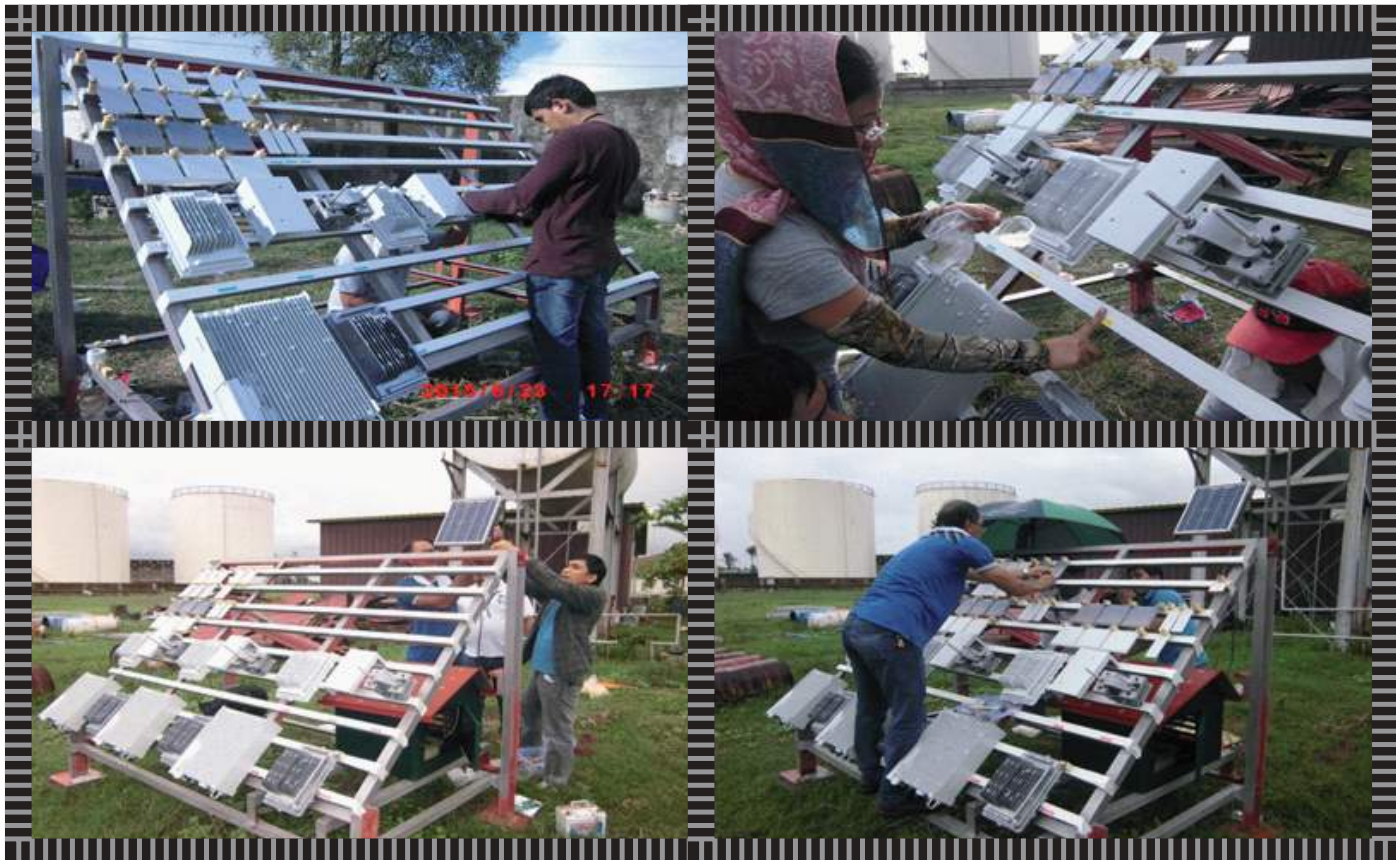
Installation of electronics equipment, installation kits and steel test panels, monitoring gadgets (temp/RH sensor, data logger, ACM sensor, and power supply), and labeling at the Marine Exposure site in Asian Chemical Corporation, Calaca, Batangas
