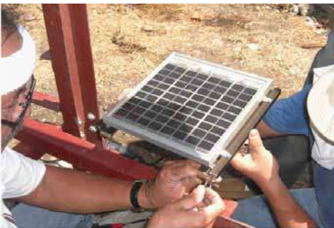
Installation of Solar Panel which will supply power to the data logger in Kemwerke, Muntinlupa
